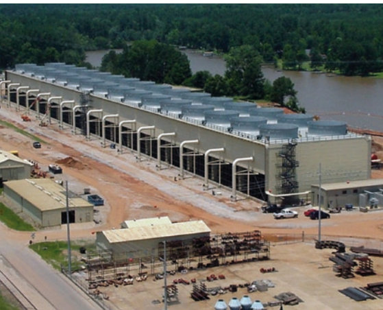
Georgia, USA 32-cell counterflow, back-to-back, fiberglass cooling tower
