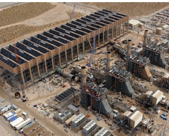
Nevada, USA 2 x 10 x 5-cell air-cooled condenser
